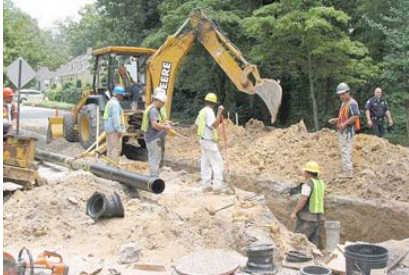
Water main replacement projects, like the Garden Hills project (completed in 2004) are under way across the City.
