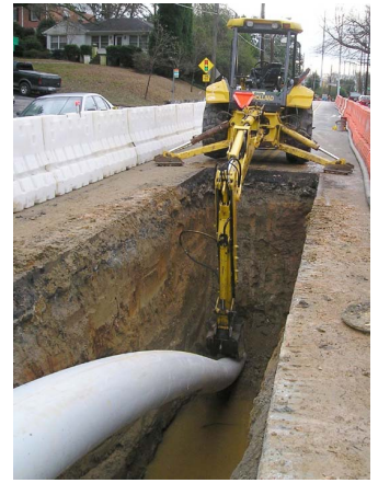
Where possible, the City is using trenchless methods of sewer rehabilitation to lessen the inconvenience to our customers.
